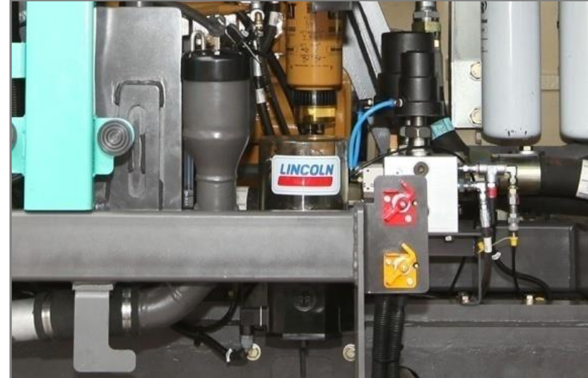
Centralized Greasing System
