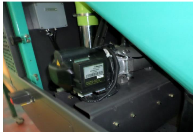
Engine Preheating System
